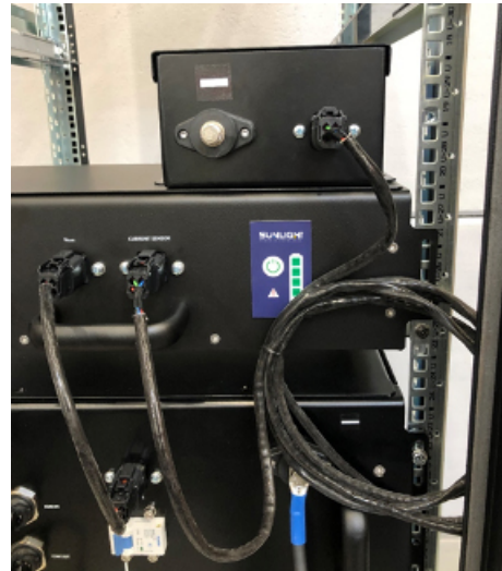
Picture 28 Shunt Box connection
