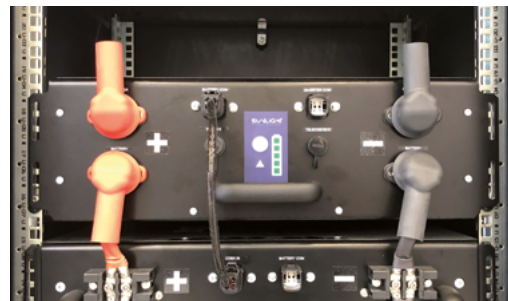
Picture 25 Li.ONESS P.U communication connection to Li.ONESS Module 1
