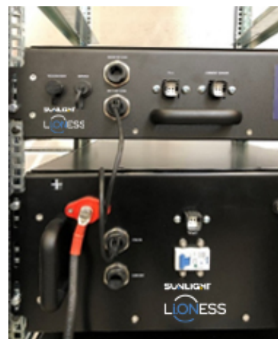
Picture 26 Li.ONESS PBT Unit communication connection to Li.ONESS Module 1
