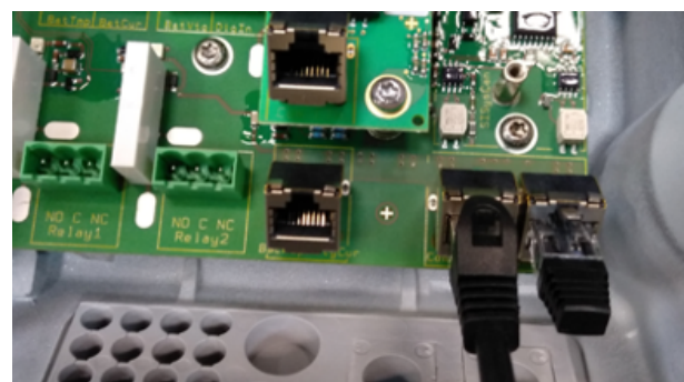
Picture A1.4 Inverter's Communication cable with the battery (Inverter's side)
