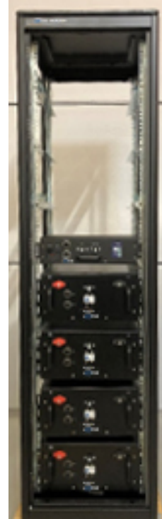
Picture 22 Li.ONESS System installed at battery cabinet
